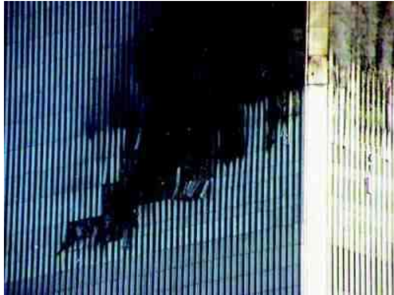
Figure 2-24 Southeast corner of WTC 2 shortly after aircraft impact.
