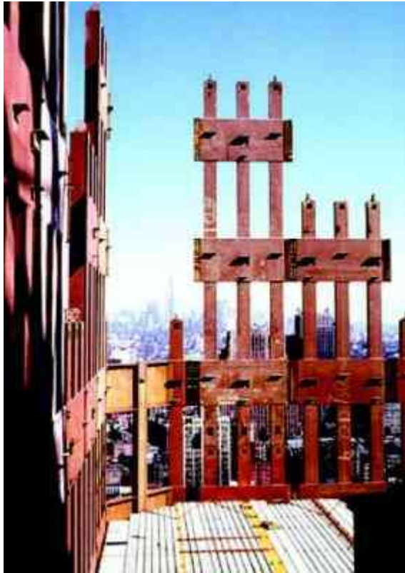
Figure 2-7 Shows the erection of prefabricated components, forming exterior wall and floor deck units.
